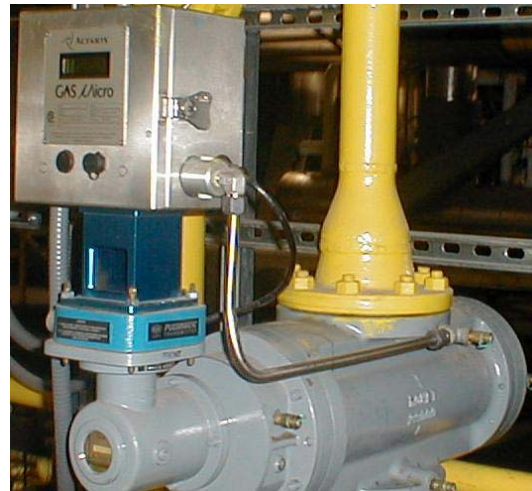
Pictured above: Rotary Meter with Pulser Installed Under the Galvanic PT Corrector
